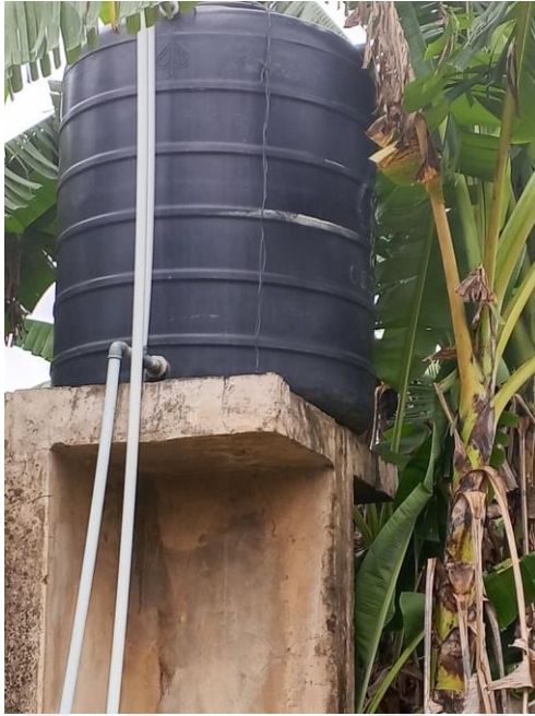
Figure 5: Overhead Storage Tank for Water Supply
