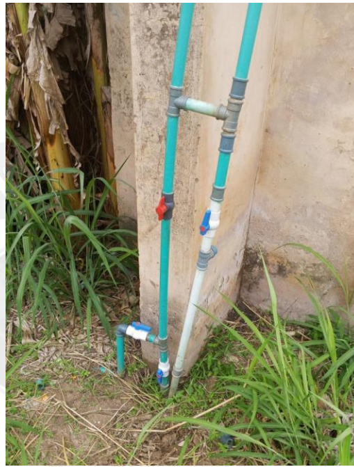
Figure 6: PVC Pipe Network
